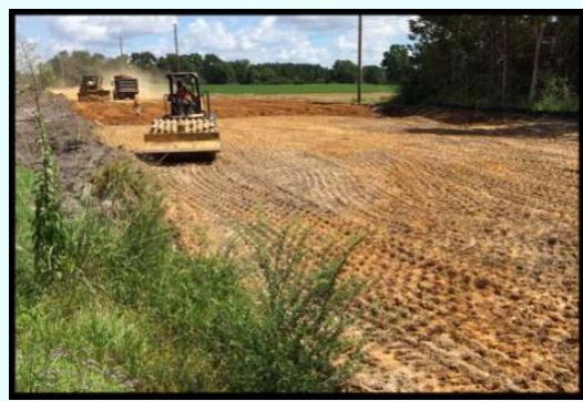
Crews continue to clear trees and shrubs, excavate and construct embankment along the 16 mile corridor.
