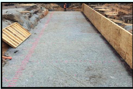
Drainage improvements are underway. Crews are working to install a box culvert south of State Park Road. This 22 x 186 foot concrete drainage structure will carry water under the new roadway to a designated drainage area.
